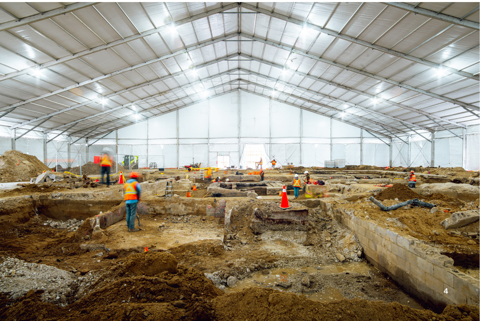
Indigenous communities conducted archaeological investigations at the site of Canada's first parliament building in Toronto during an early phase of the Ontario Line.
