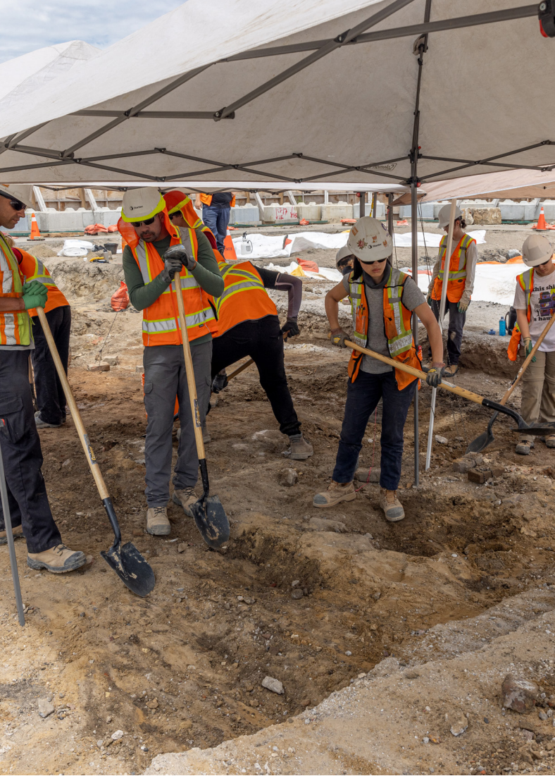
Indigenous communities conducted archaeological investigations at the site of Canada's first parliament building in Toronto during an early phase of the Ontario Line.
