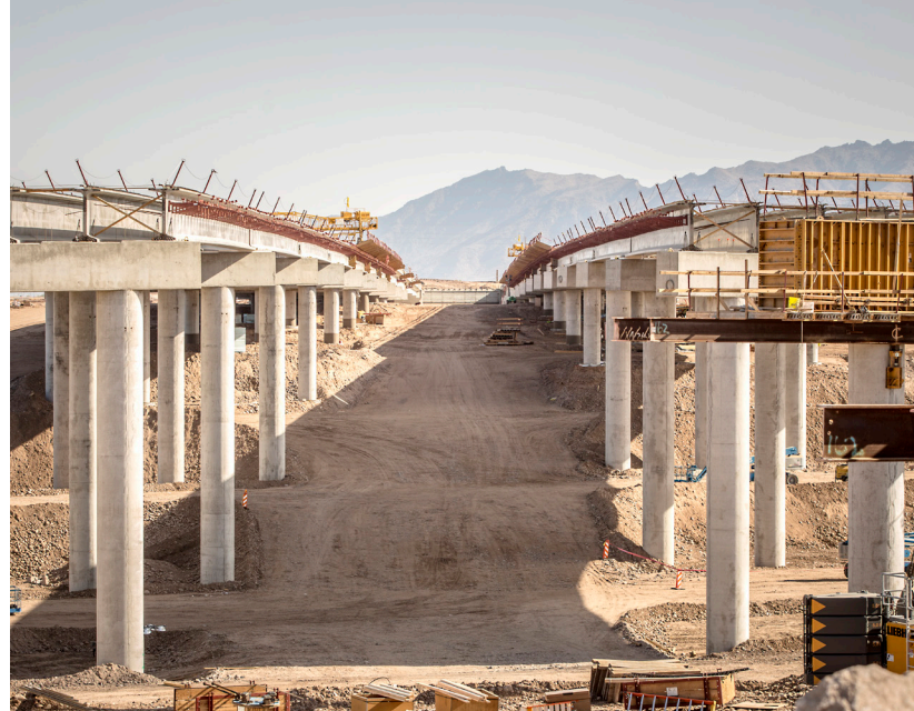
The South Mountain Freeway project in Arizona, delivered through a public-private partnership.
